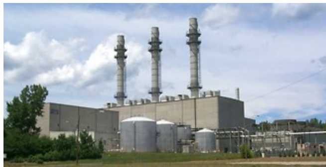
Maxim Power's Pittsfield, Mass., generator. (Source: Maxim)
